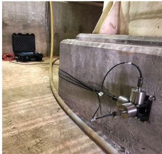
Installation SVi minimate pro accelerometer
