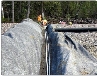
◆ Shape Accel Array (SAA) installation in horizontal orientation
